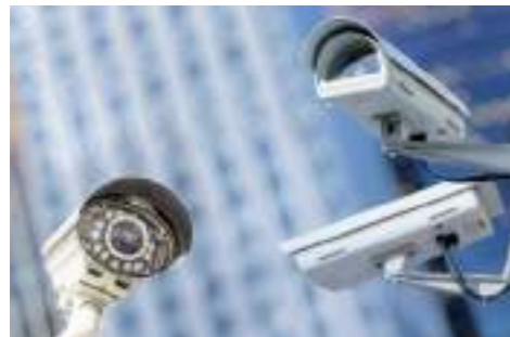
CCTV System for Streets
