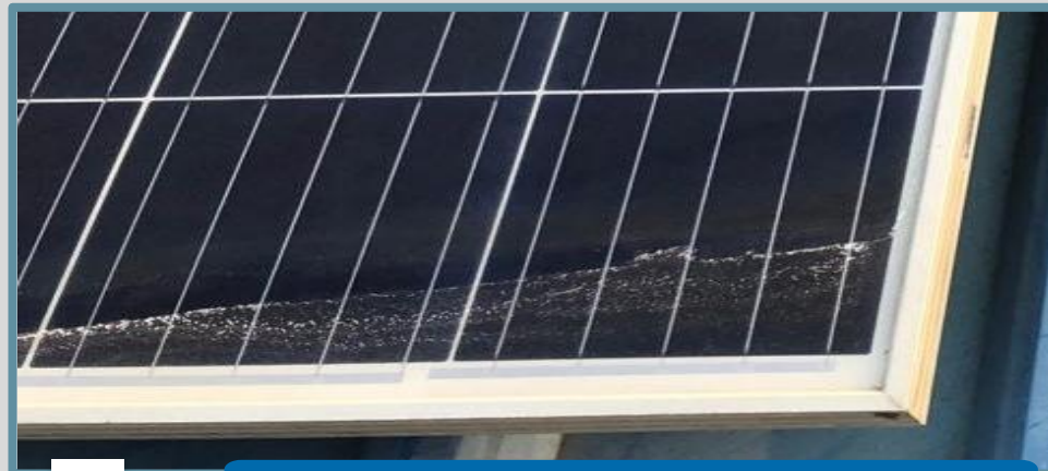
03 Residual stains after water cleaning
