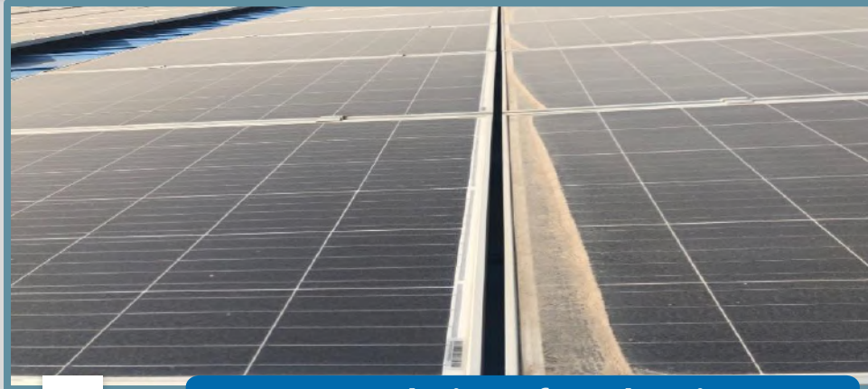
01 Dust accumulation after cleaning one month later
